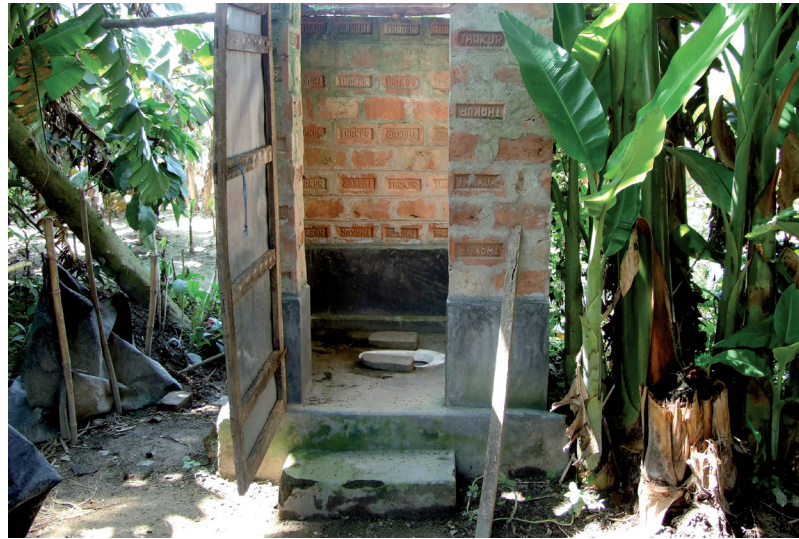
Brick-walled latrine, fully funded by the benefiting household, Kolkatta
